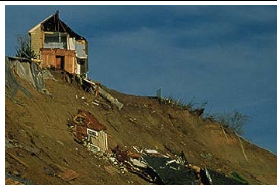
Landslides can damage or destroy roads, railroads, pipelines, electrical and telephone lines, mines, oil wells, buildings, canals, sewers, bridges, dams, seaports, airports, forests, parks, and farms. (Photo by Lynn Forman)
