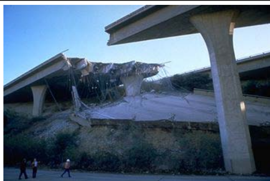
Many roads, including bridges and elevated highways, were damaged by the 6.7 magnitude earthquake that impacted the Northridge, California area January 17, 1994. Approximately 114,000 structures were damaged and 72 deaths were attributed to the event. Damage costs were estimated at $25 billion. (FEMA News Photo)
